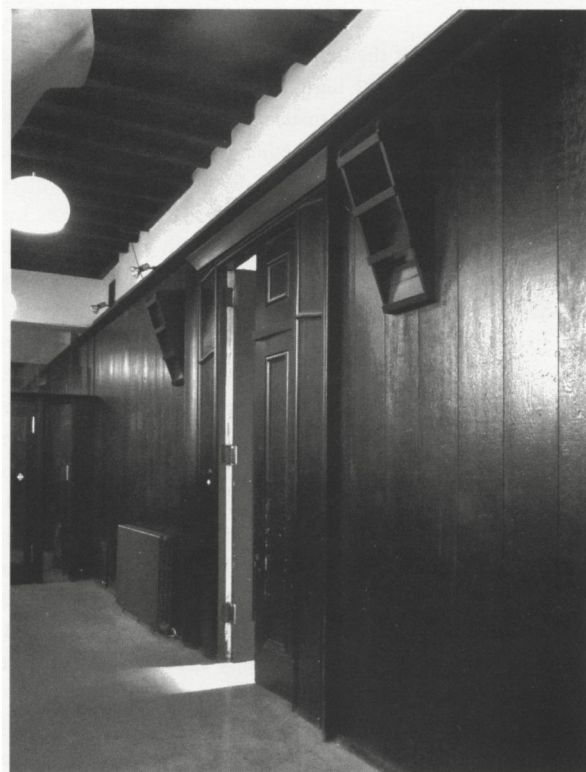
Figure 16. Closed ventilation drawers on the spine wall, ground floor corridor. (Image: Ranald Lawrence)
