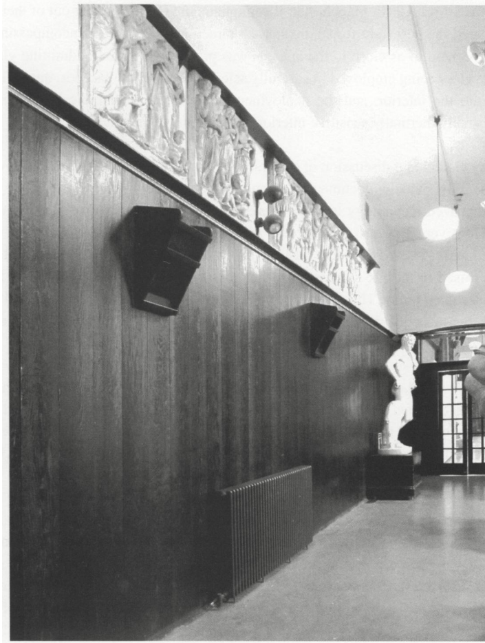
Figure 17. Open ventilation drawers on the spine wall, first floor corridor. (Image: Ranald Lawrence)
